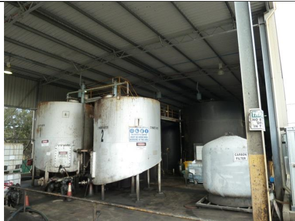
Photo 1: Tank Farm – Tanks 1 and 2 and Carbon Filter used for sewer discharges
