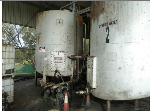
Photo 2: Tank Farm – Tanks 1 and 2. Drainage also noted beneath tanks
