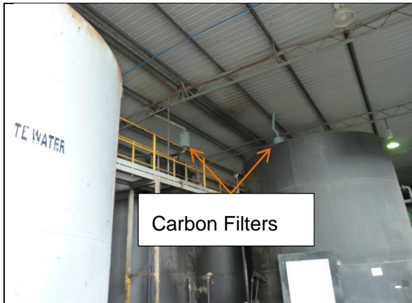
Photo 7: Activated carbon filters connected to Tanks
